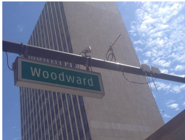
Arada Systems, Inc. Roadside Units on Woodward Avenue in Detroit on Traffic Pole
